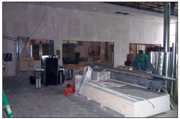
This is a view looking toward the kitchen from the dining room. The large window is the serving line.
